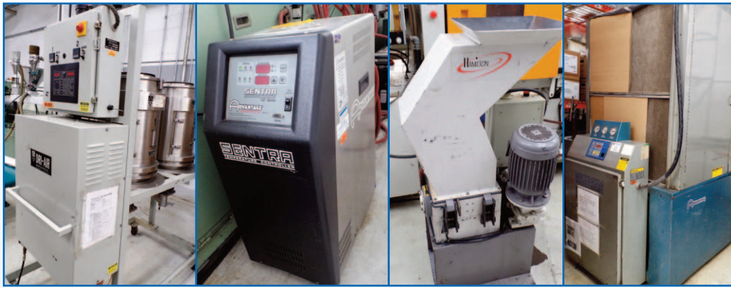
PARTIAL VIEW OF PLASTIC SUPPORT EQUIPMENT
